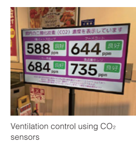
Ventilation control using CO2 sensors
