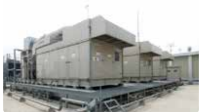
Aeon's private power generators
