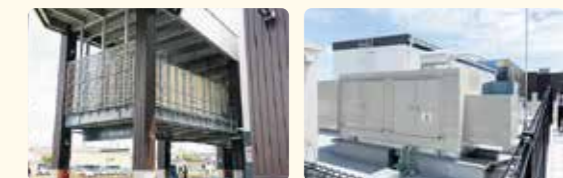
Vital equipment, such as water tanks, emergency generators, and electrical substations, are located out of reach of expected water levels.
