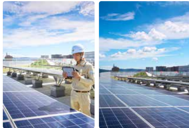
Aeon Fujidera SC Inspections by facility managers and use of cutting-edge technologies to achieve efficient facility operations
