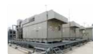
Aeon's private power generators
