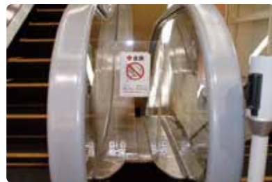
A safety measures for escalators
